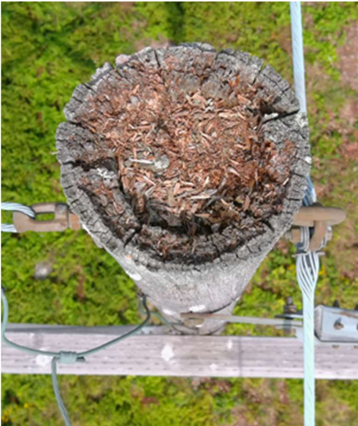
Structure 212 – Pole Top Rot & Rusted Hardware
