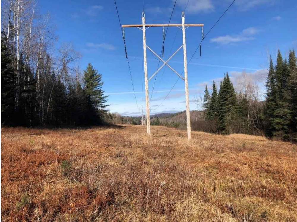
Photograph No. 53: Looking northerly at proposed access and work pad location for Structure 348.
