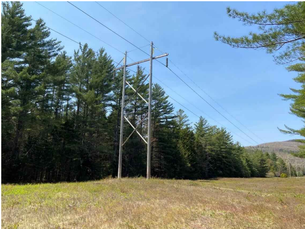
Photograph No. 18: Looking westerly at proposed access and work pad location for Structure 297.
