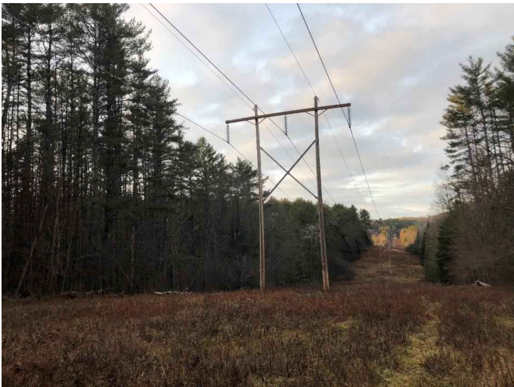
Photograph No. 70: Looking northwesterly at proposed access and work pad location for Structure 365.
