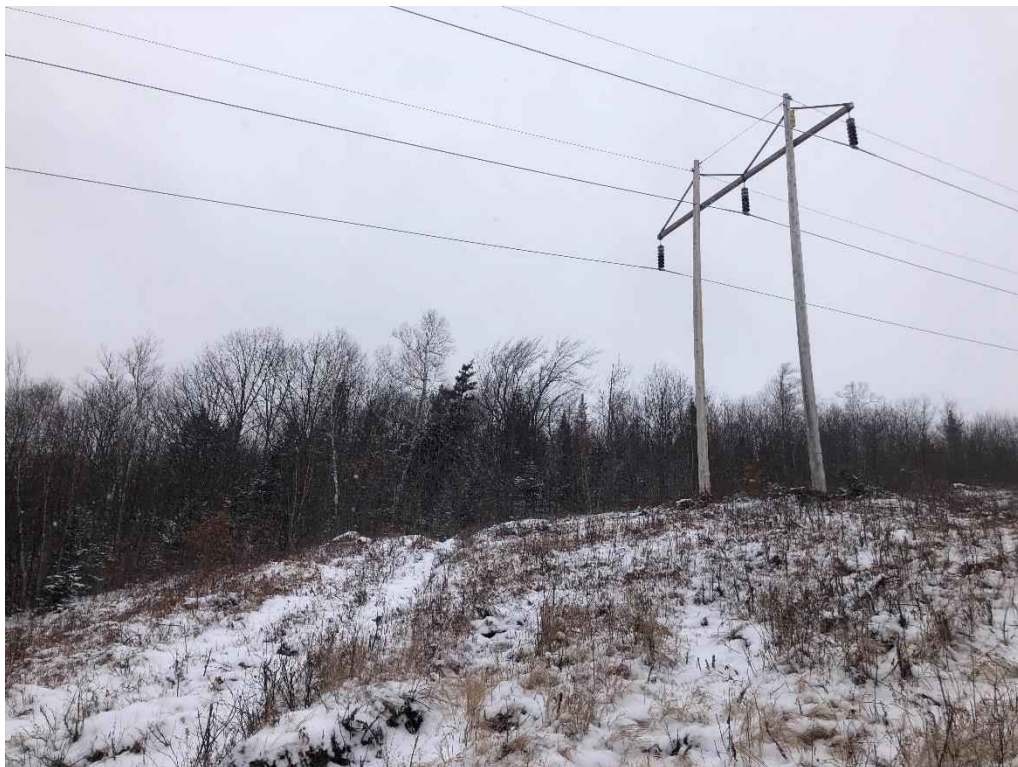
Photograph No. 28: Looking southeasterly at proposed access and work pad location for Structure 322.
