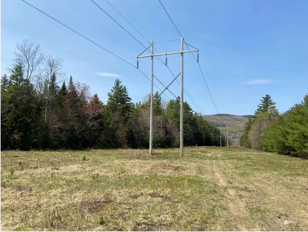
Photograph No. 17: Looking westerly at proposed access and work pad location for Structure 294.
