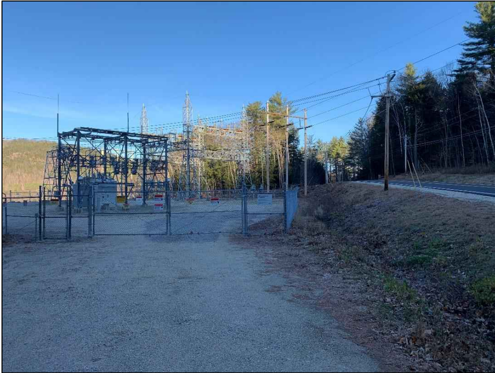
Photograph No. 1: Looking westerly at Structure 170, located within the Woodstock Substation.
