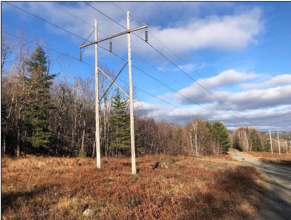
Photograph No. 50: Looking northwesterly at proposed access and work pad location for Structure 344.
