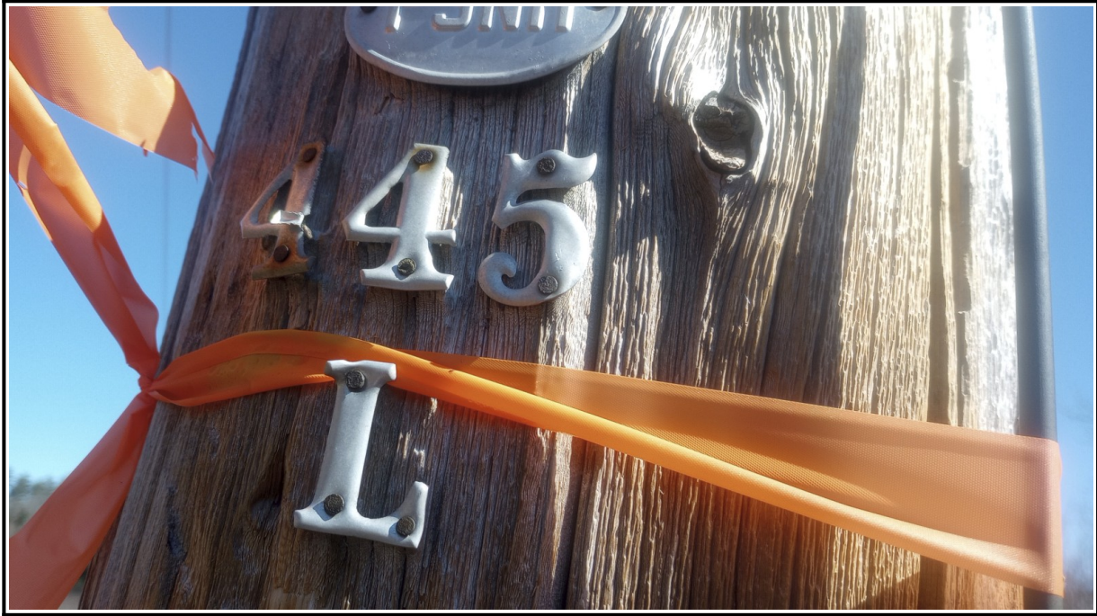
Pole on the Streeter Pond tap to Whitefield (1969) section of the X-178:
