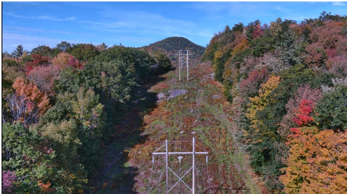
Photograph 4: View north of ROW between Existing Structures 119 (foreground) and 120 (in the distance). Bedrock outcrops and boulders can be seen south of 120.
