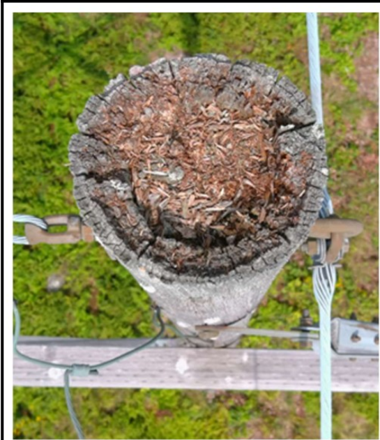
Structure 212 – Pole Top Rot & Rusted Hardware
