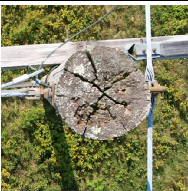
Structure 356 – Split Pole Top
