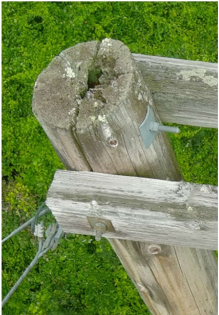
Structure 25 – Pole Top Rot and Splitting at Hardware Attachment Point
