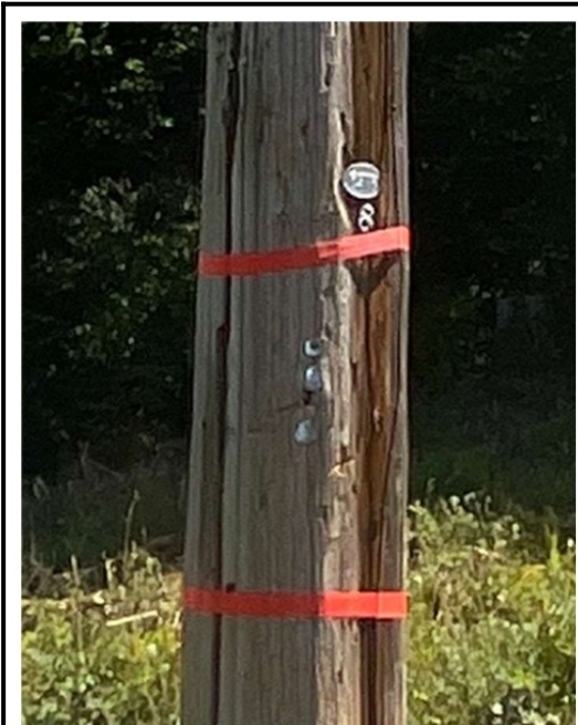
Structure 8 – Severe Structure Splitting
