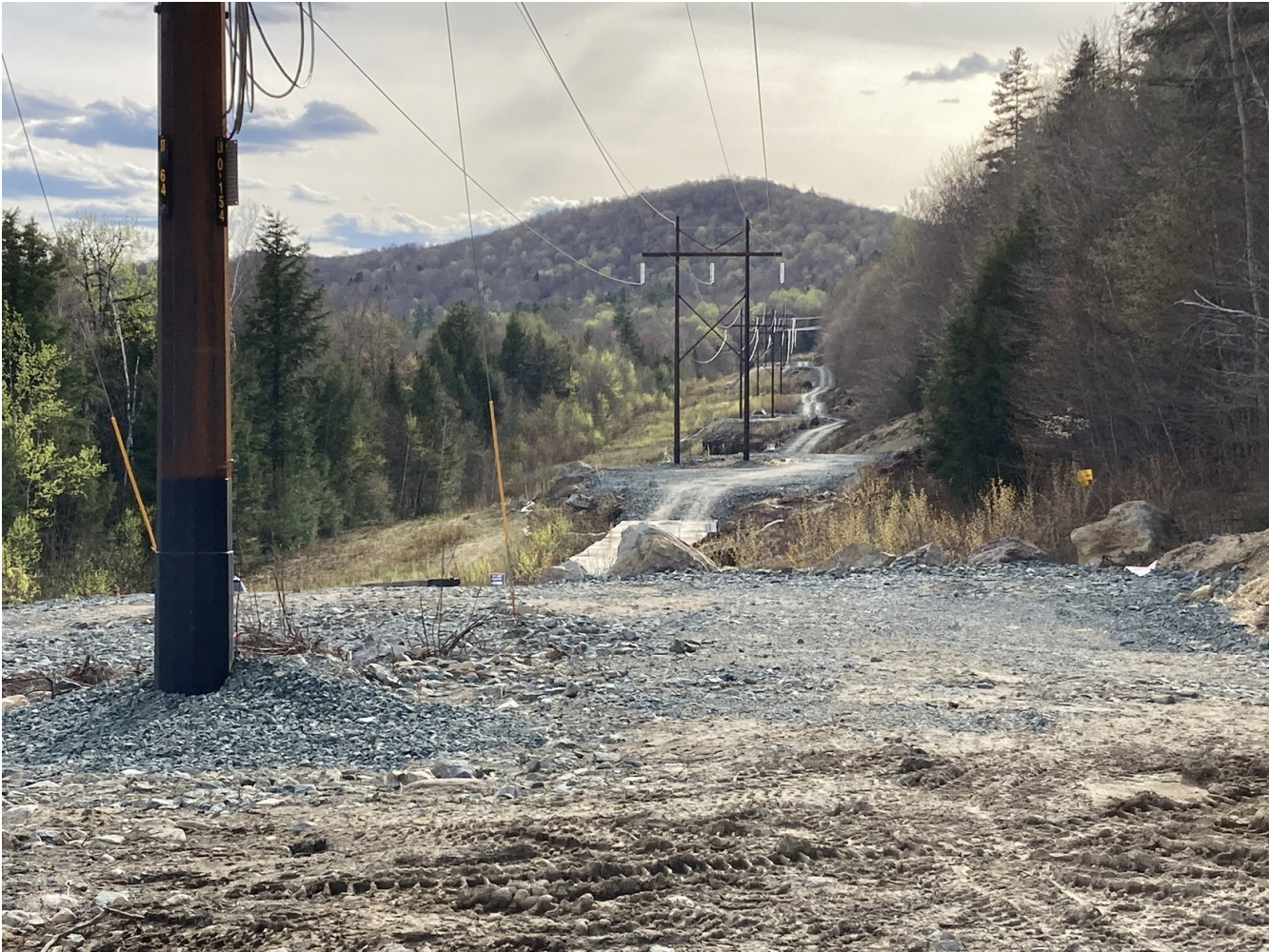
O-154 line after “upgrade”, with “enhanced” roads.
