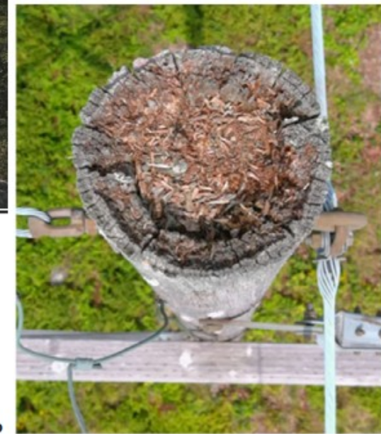
Structure 212 – Pole Top Rot & Rusted Hardware
