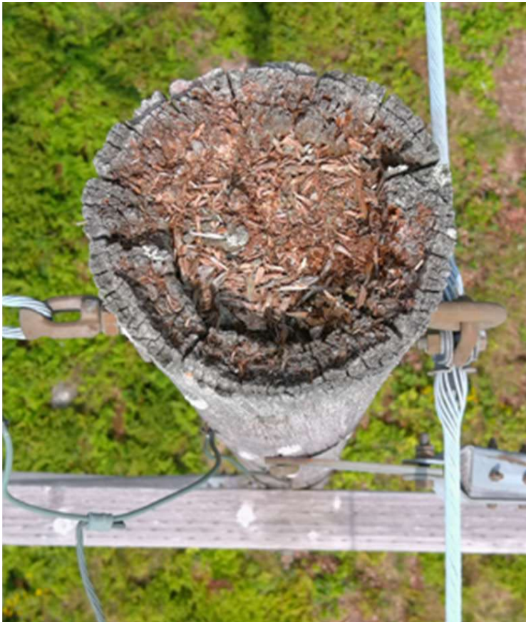
Structure 212 – Pole Top Rot & Rusted Hardware
