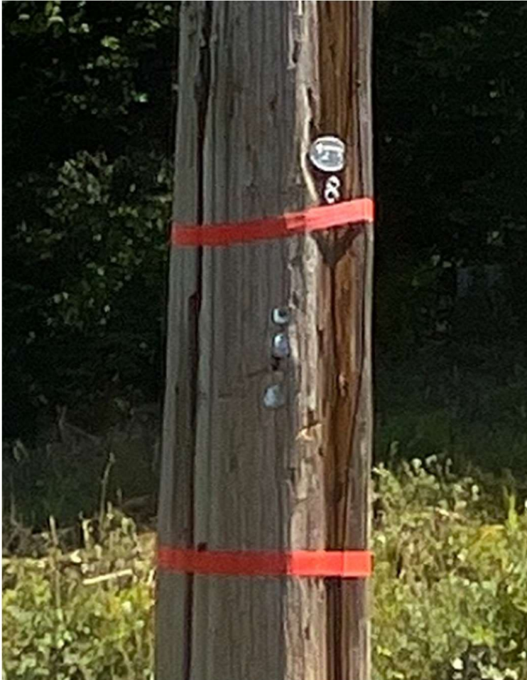
Structure 8 – Severe Structure Splitting
